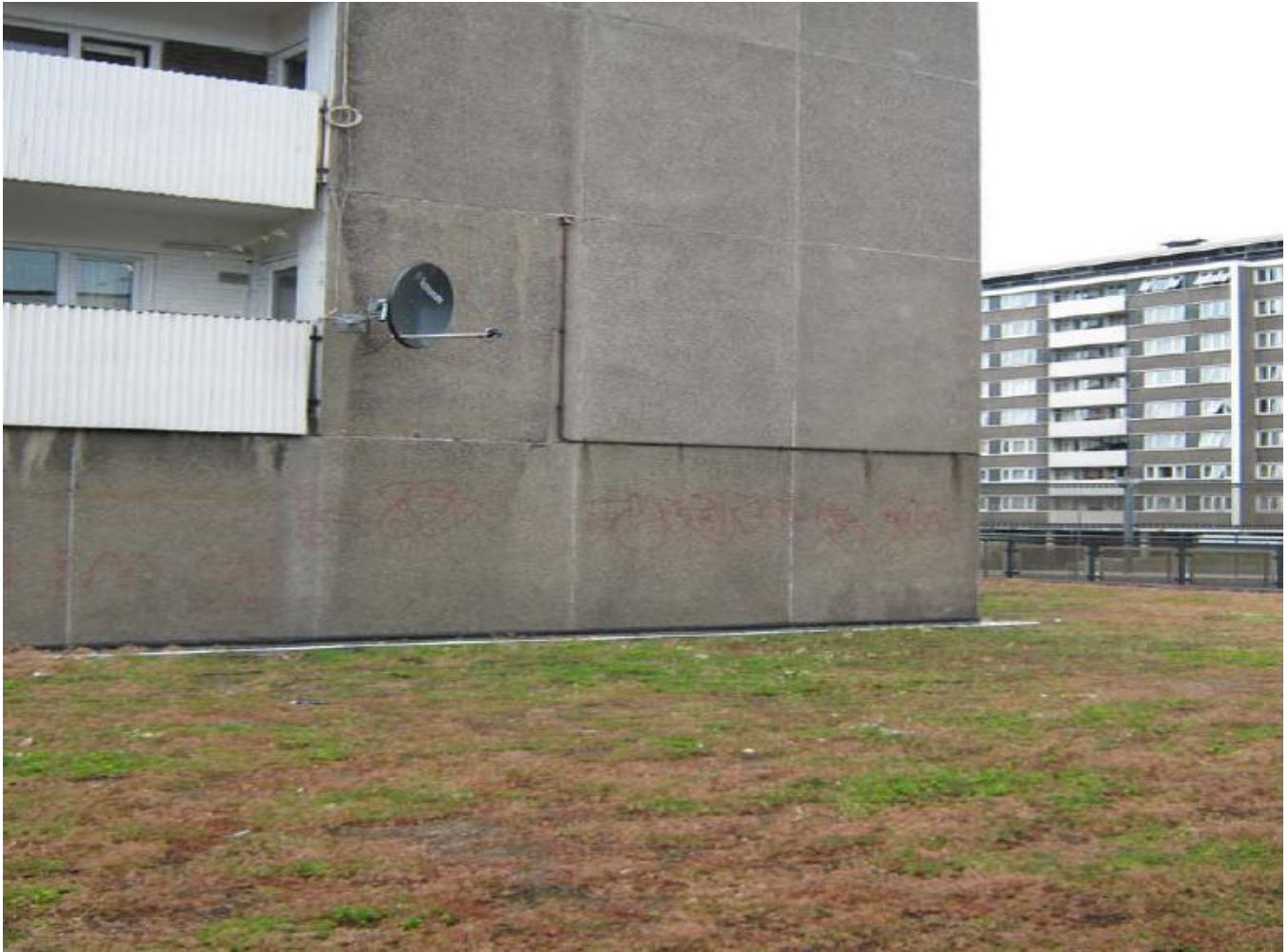
Image 3: Ground floor side elevation of Michael Cliffe House facing south with Patrick Coman House in the background.
